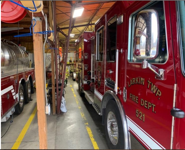
Photo: Left Side of engine bay between Tender 520 and Engine 521
